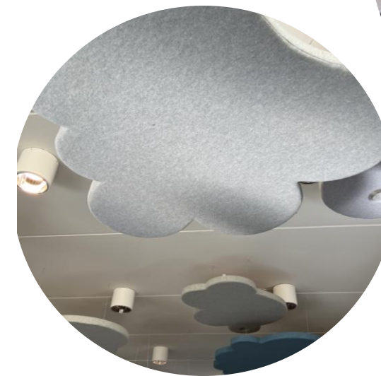
Figure 10. Acoustic panels reducing noise in the ceiling- Rauma teacher training school @Anna Laukkarinen
